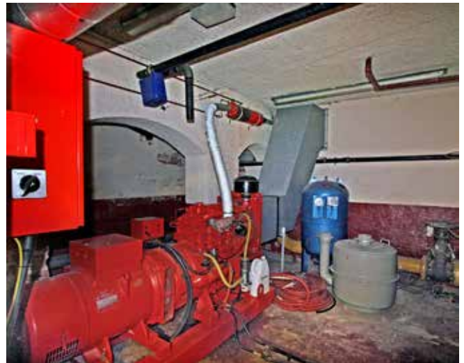
Emergency generator. A filter drum is sitting on the floor
